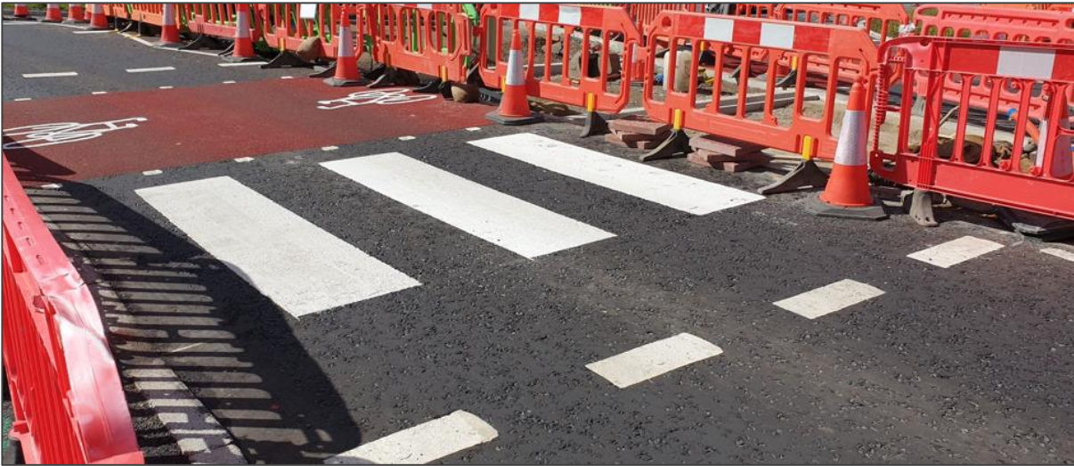
New parallel crossing being constructed at the south end of Alexandra Road
