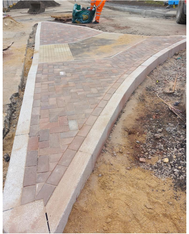
(Old) Lynchford Road - New traffic Island installed with block paving and tactile paving
