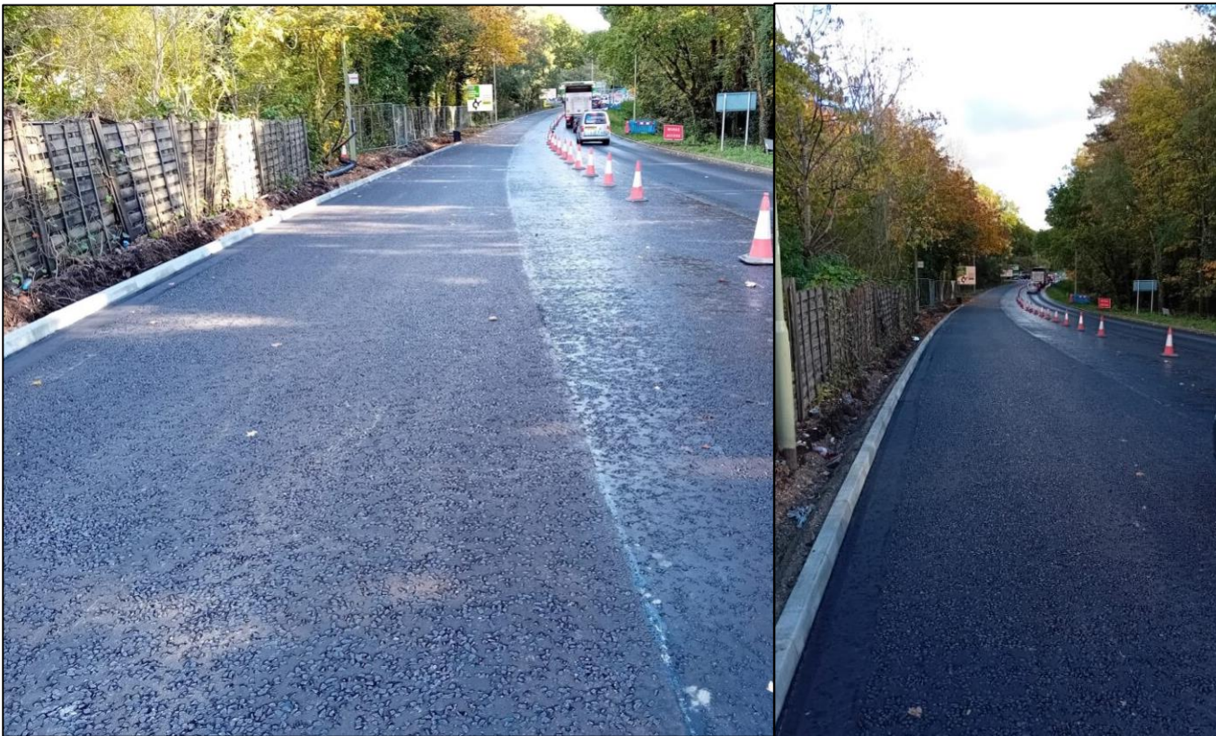
Completed surfacing works looking east from Artillery Road towards Park Road roundabout. This will provide two permanent eastbound lanes on the approach to the roundabout to ease congestion.
