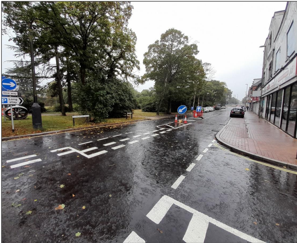
Lynchford Road – Re-surfacing has been completed on the section between Camp Road and Old Lynchford Road.
