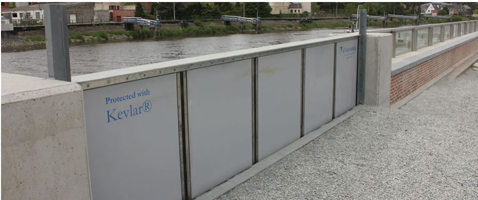
Typical Flood Gate
