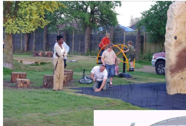
Hollybank Park installation, Emsworth
